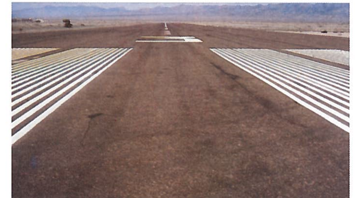
Reclamite preservative seal was applied to this ten-year-old asphaltic concrete pavement runway. Due to the dry, brittle pavement condition, total absorption of the Reclamite eliminated the need for sanding.
