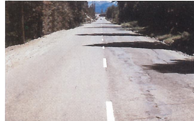
Reclamite was applied to the left-hand lane; the right-hand lane was not treated. This photo, taken five years later, shows severe distress, requiring patching and maintenance. The Reclamite-treated side (left) shows no distress and requires no maintenance.
