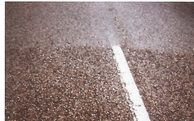
Reclamite was applied to the upper portion of this open-graded pavement; the lower portion was not treated. This photo, taken four years after application, shows severe loss of aggregate in the lower untreated area. The upper Reclamite-treated portion shows no surface loss or distress.
